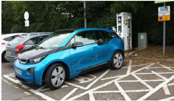
May 2018 - PivotPower announces plans to build 2GW of batteries with EV charging, also to provide new 'flexibility services' to the SO
