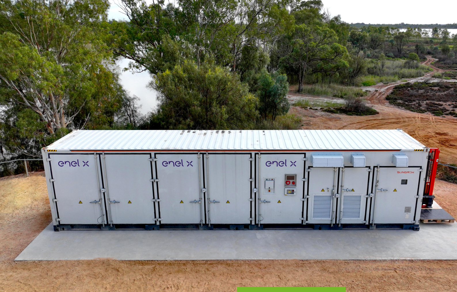
© ENEL X BESS, Barmera, South Australia
